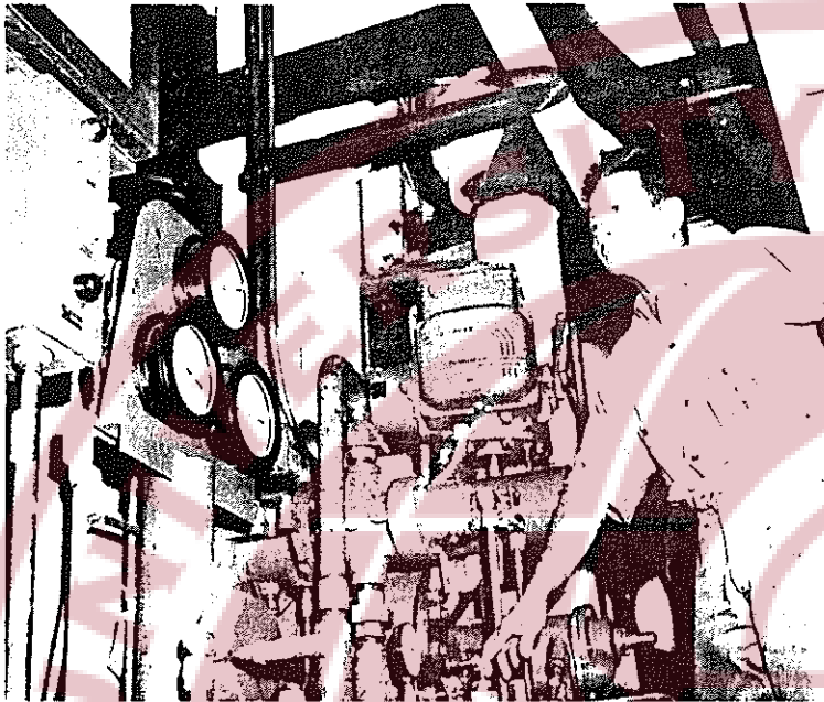
Feliciano Galiza checks on another duty of engine tender mechanics, operating the turbine. Two men are on this job each shift. Those not pictured here are Hirotsuke Oshita, Frederico Tonogan, Antonio Castillo, James Gabuco and Andres Pagdilao.
