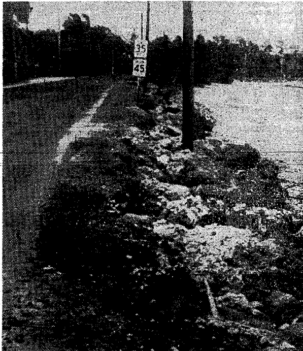
THIS STRETCH OF territorial highway at Punaluu is marked off with caution signs for safe and slow driving but as the picture shows, present danger comes from its narrow shoulder. Large cracks are on the roadside and waves are washing it away. Some Punaluu residents say that if the shoreline, especially the mouth of the Punaluu stream is dredged, the damage to the road by waves can be lessened.
