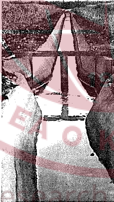
NO WATER LOSS with concrete lined ditches. Crayfish and water seepage are hard on dirt ditches. This new ditch carries wash water from the cane cleaner to fields below the mill. Concrete helps put the water in the fields where it belongs without waste.
