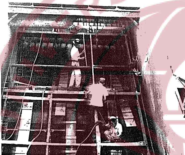
Torajiro Sato, fireroom foreman, looks on while the bricklayers from Pell & Company put the finishing touches on the number five boiler.
